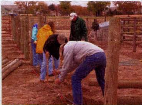
Make a Difference Day brought many volunteers to the Bee Farm, where they helped construct corrals.
